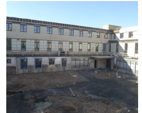
La construction de la ressource intermédiaire progresse Construction of the Intermediate Resource in progress
